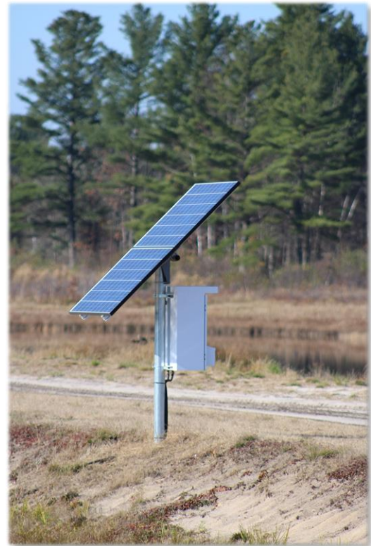
Pole-Mounted, Permanent Install Shown
